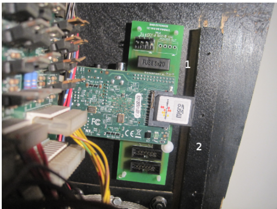
Figure 7 – Mounting location close up
