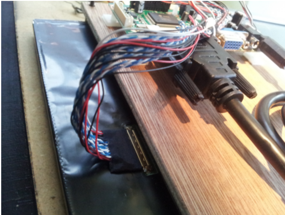
Figure 7 – LVDS cable connected to the LCD panel
